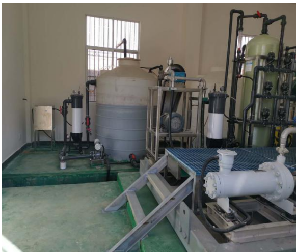
渗滤液处理药剂箱
